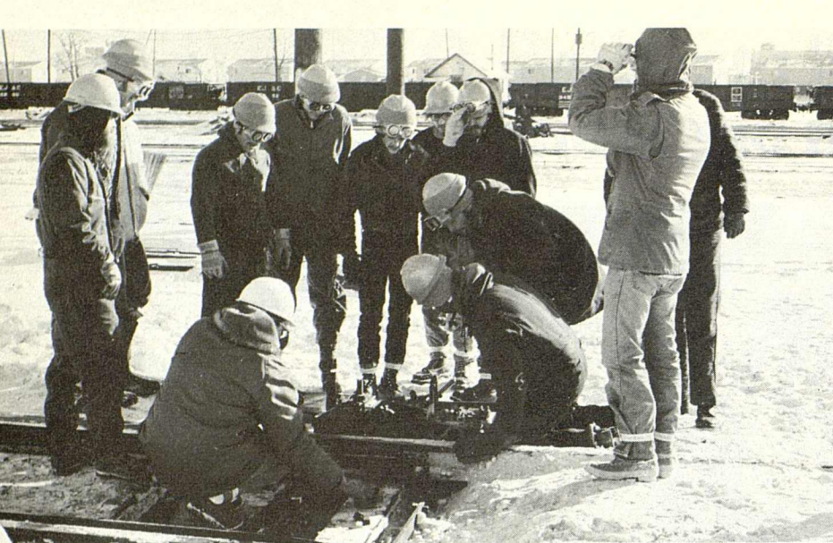
A class at the new System Training Center at Columbus, Ohio, installs lock and point detector rods in switch on training track.
